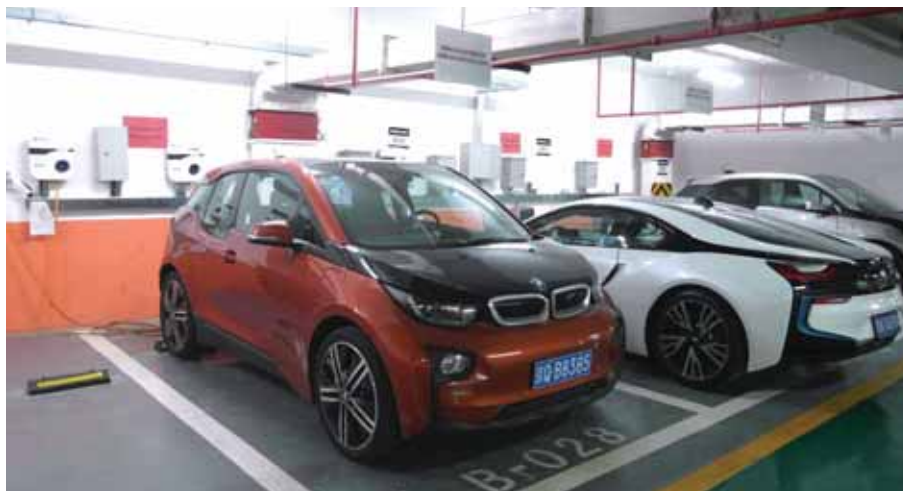
Charging stations installed at Gateway Plaza's car park encourage tenants to use eco-friendly vehicles.
