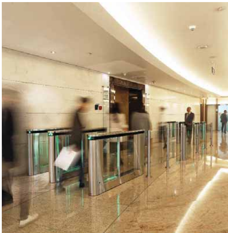
New security turnstiles and lift-access card control system at Gateway Plaza.
